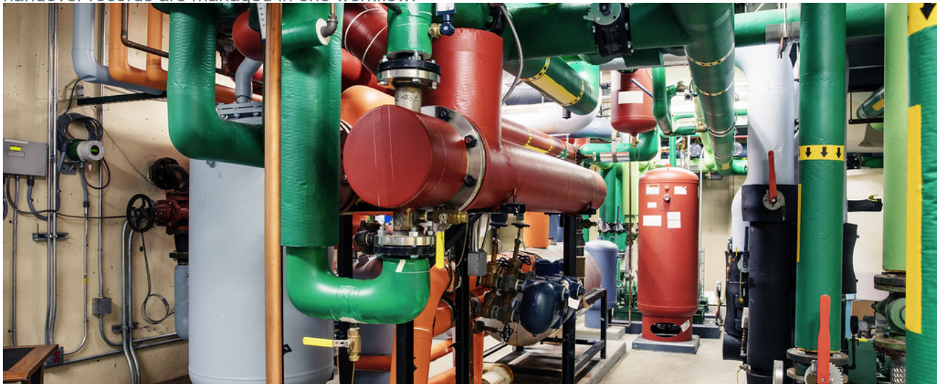
Plant rooms, boiler rooms and industrial piping
